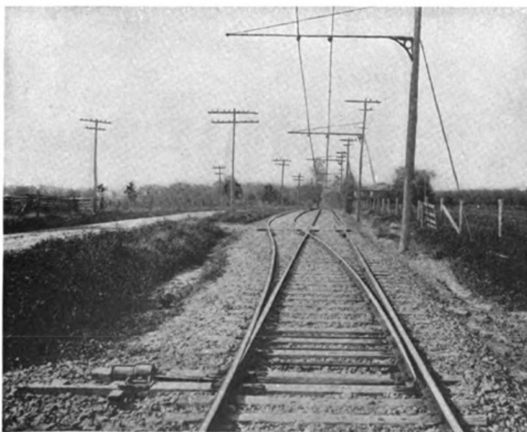
TYPICAL SWITCH, WESTERN OHIO
