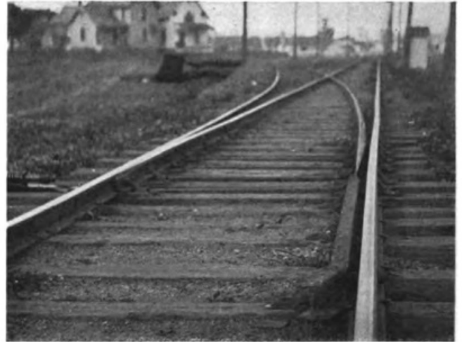
PROTECTING GUARD-RAIL AT SPRING SWITCH POINT, STARK ELECTRIC
